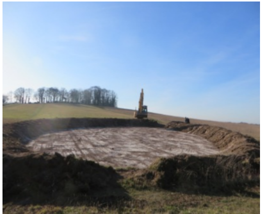
The new scrape on North Down in January 2020. The digger completes the shaping of the banks.
