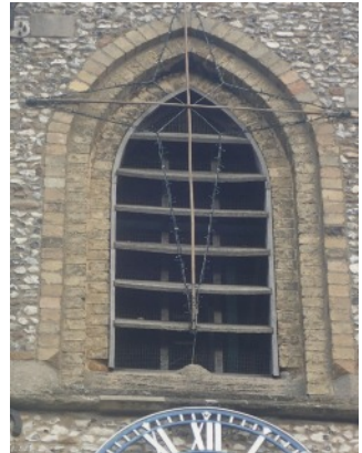
Tower south belfry window: C14 Barnack sill below 1803 Gault brick jambs and arch, probably replacing C14 Clunch
