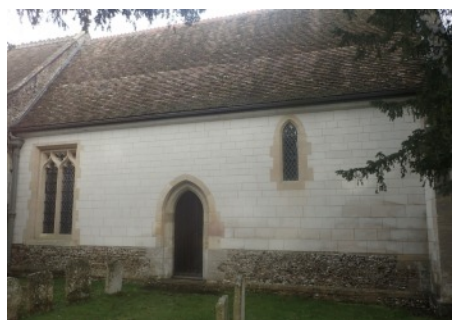
Chancel: C20 Portland Whitbed ashlar wall replacing C13 local Clunch, over fieldstone/flint rubble plinth. Windows mostly C20 Clipsham repair. Door with C13 Barnack plinth and Clunch inner jambs then possible 1873 Casterton repair of outer jambs and arch
