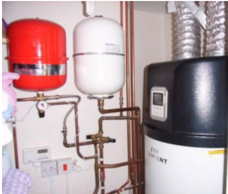
Our airing cupboard showing the EAHP (right)
